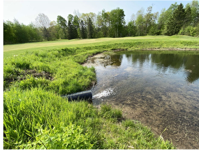
Photograph 10: Perched culvert at inlet to Pond #15 along Tributary A (May 23, 2023).
