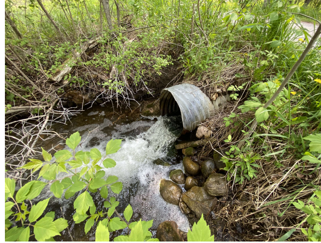
Photograph 6: Perched culvert at upstream limits of property along main branch of Silver Creek (May 23, 2023).
