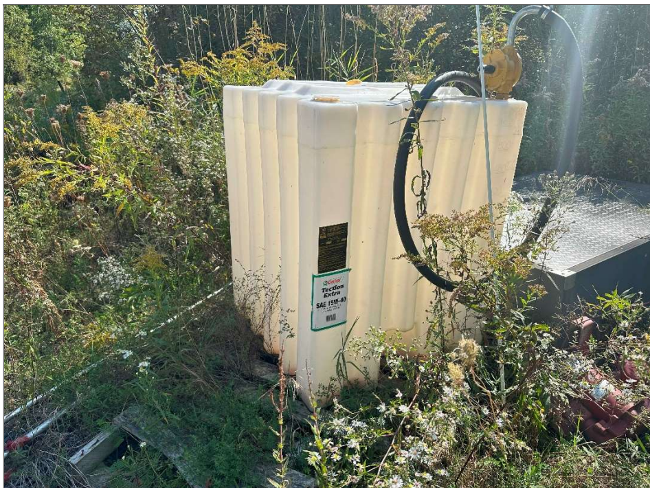
Photo 40 – Empty oil tank in the derelict equipment storage area.
