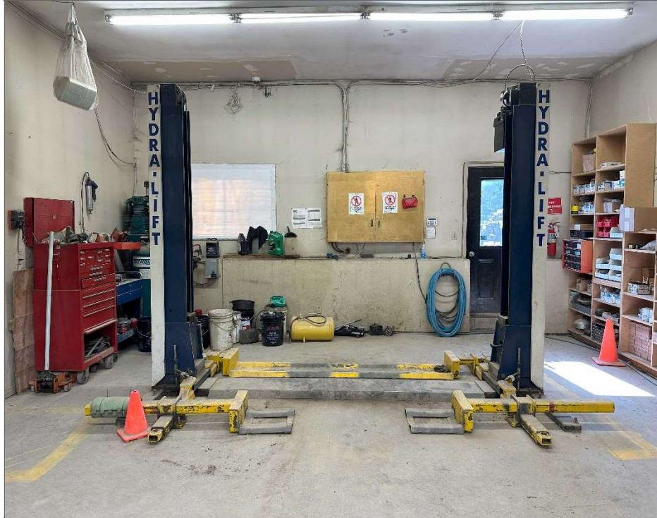
Photo 21 – Automotive hydraulic lift located in the southwest of the maintenance building, view southwest.
