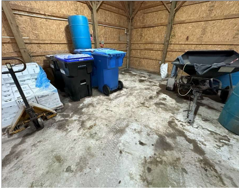
Photo 31 – Recycling bins and chemical pallet surrounded by staining and absorbant on the floor of the northern corner of the maintenance building, view north.
