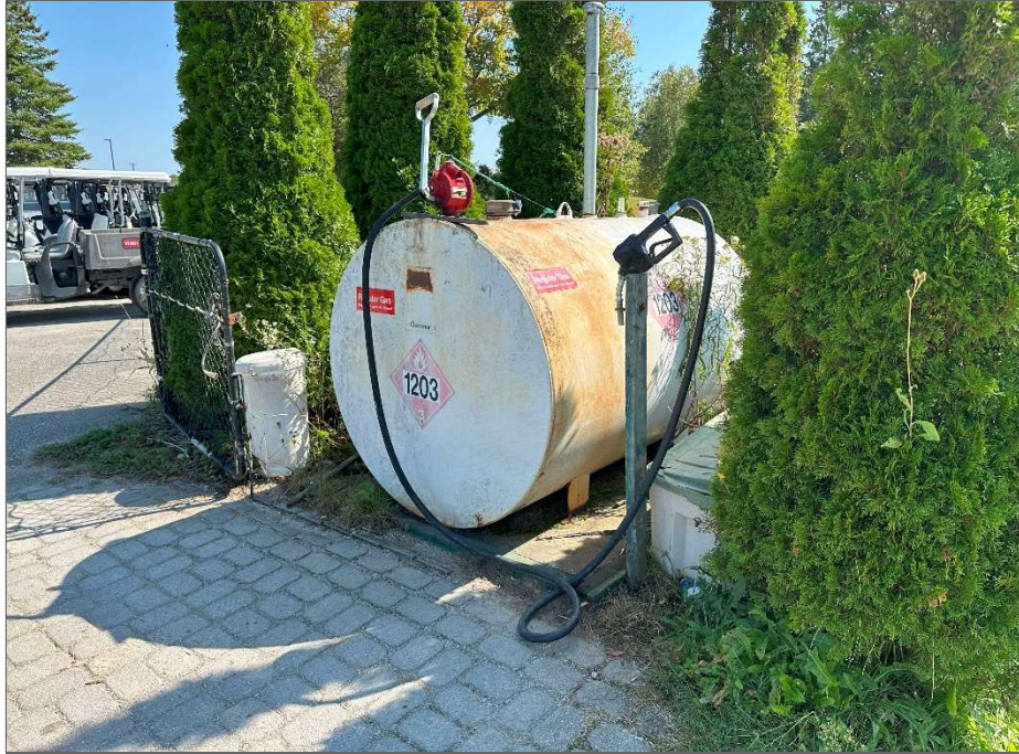
Photo 13 – 2200 L aboveground storage tank (AST) west of the golf cart storage lot, view southeast.
