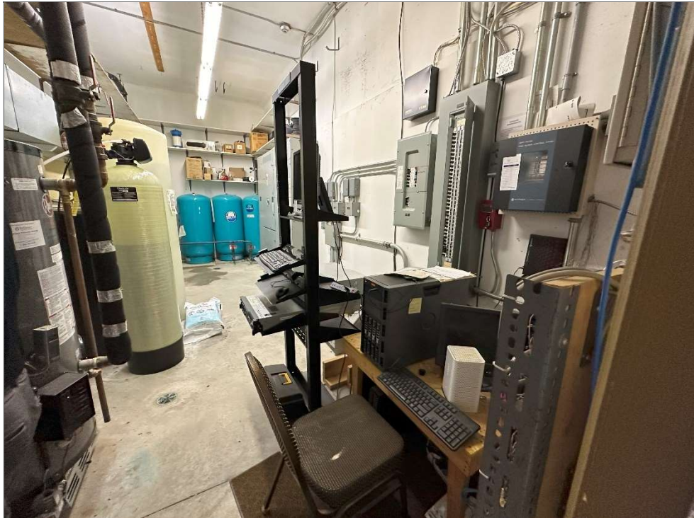
Photo 10 – Clubhouse electrical room, looking northeast.
