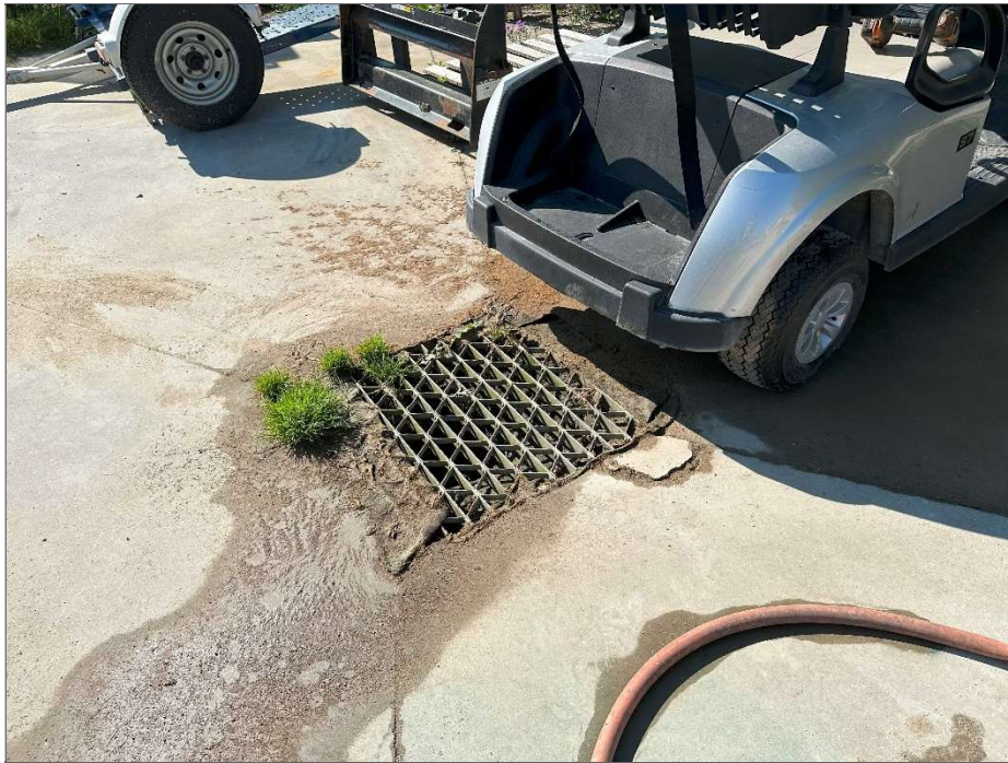
Photo 38 – Decommissioned/blocked drain in the spill capture area.
